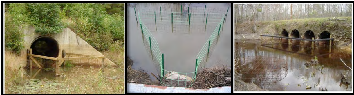
Figure 43: Examples of culvert-protective fences. From left to right: (a) and (b) are stand-alone culvert-protective fences, while (c) is a stand-alone fence combined with a flexible pond leveler pipe (underwater and not visible) and a cylindrical wire mesh cage, which provides extra protection against obstruction. Figures from Boyle (2006).
