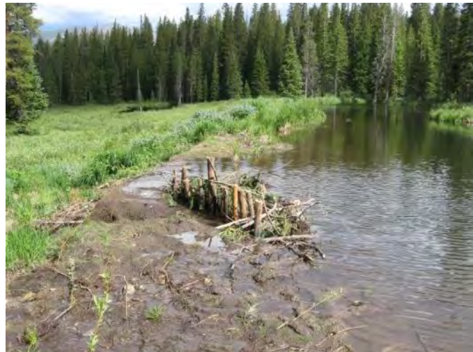
Figure 68: A PLWW was constructed on one repaired dam to temporarily fortify a nick point while we were waiting for beaver to reoccupy the site
